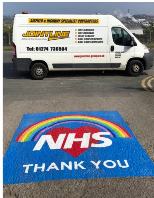
Jointline Ltd and FORS associate Dawes Highway Safety showed appreciation during the pandemic with 'Thank you NHS' road markings and design panels.
